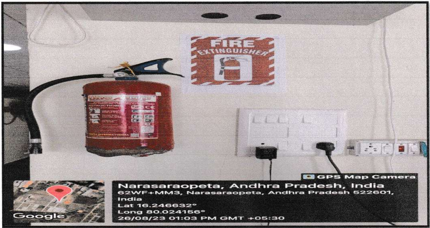
Fig: VDC has well established Safety Fire Extinguisher
