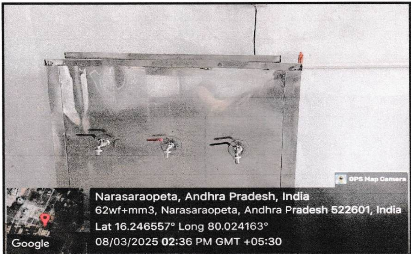
Fig: Drinking Water Facility and cooling fridge
